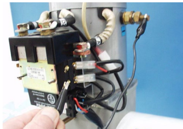
Jumping ground to blue on D2 coil
